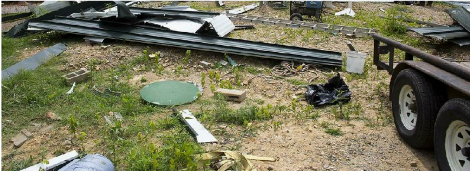
Roofers with CWR Contractors work on a restroom facility at Pinnacle Mountain State Park on Wednesday. Construction had been halted for months because of issues with a previous contractor. - Photo by Melissa Gerrits
